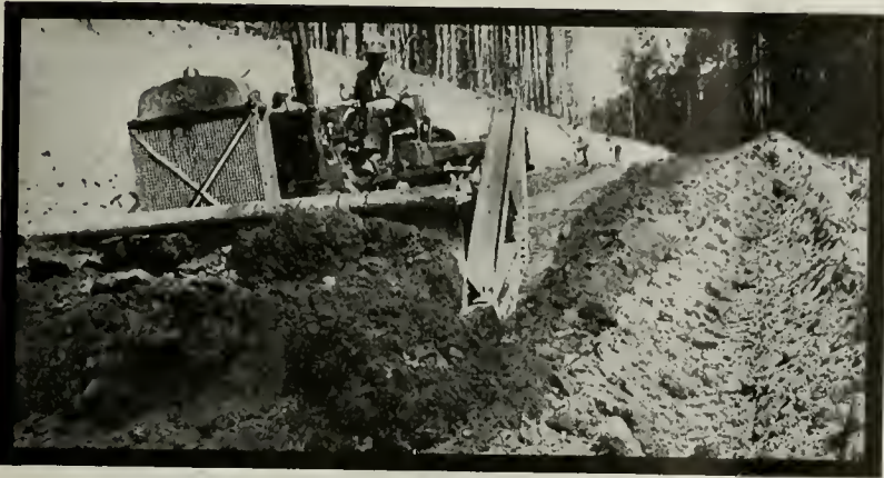
Johnson Brothers had this job on the Santiam Highway, 47 miles from Albany, Oregon
